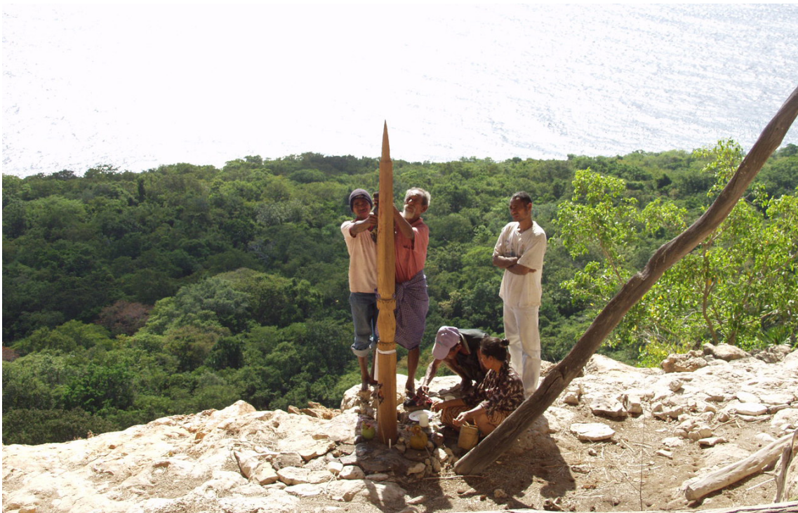
Figure 8. Ceremony following the replacement of a new téi post at Ili Kérékéké .
